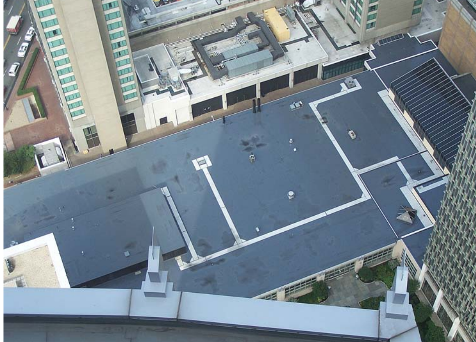
Color was a consideration when selecting a roof for The Shops at Prudential Place due to the high visibility the roof received from the surrounding high rise buildings and towers.
