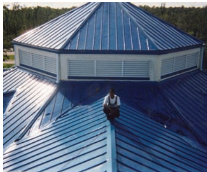
A worker gives the Hancock Medical Center's handsome, new roof a final check following installation.
