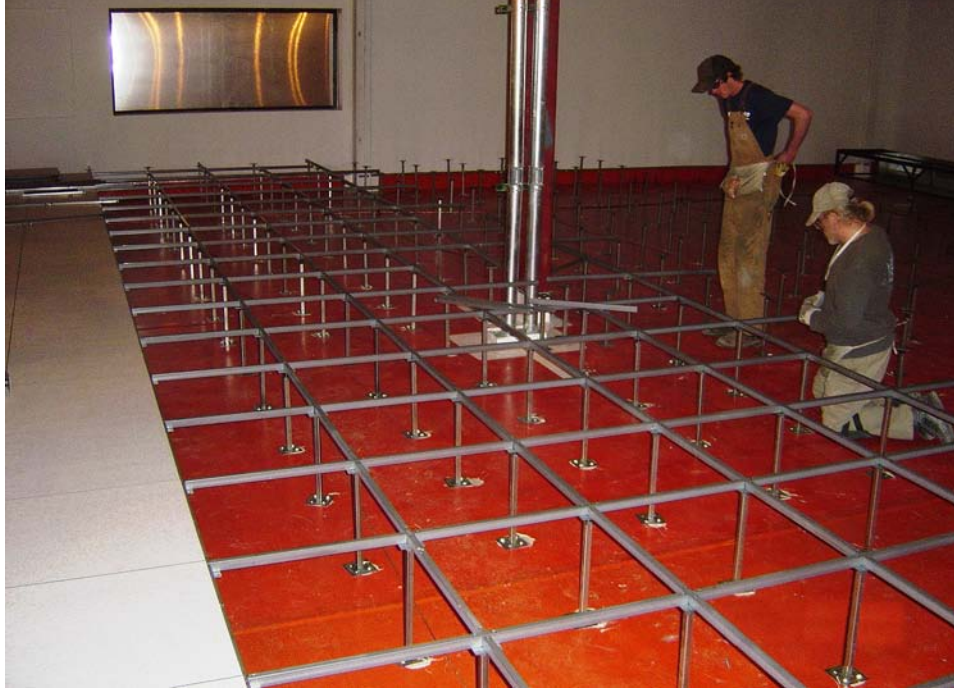
A grid system is installed on pedestals over the Sarnafil G476 membrane. To the left of the photo are floor panels, already installed.
