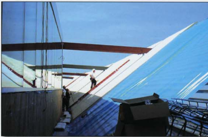
About half the roofs on the terminal are a 5:12 slope, about 25 percent are a 10:12 slope — almost a saw tooth. The balance is flat.
