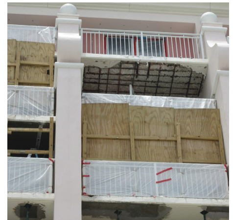
Plywood protection for rain water damage
