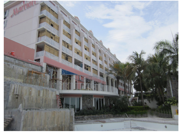
A structure needing repair
