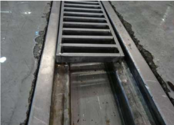
Flaws in the floor drainage connection
