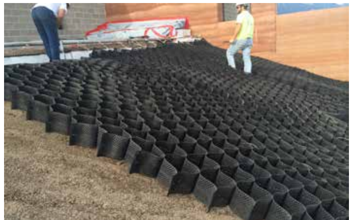
GardNet® used to stabilize LiteTop® media layer on sloped roof - Brinton Museum - Brinton, WV
