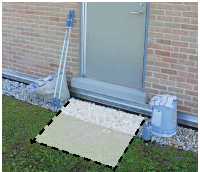
Landing pad needed at door
