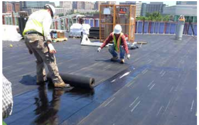
Installing Hydroflex protection sheet (RB II or 30) into second layer of MM6125 membrane
