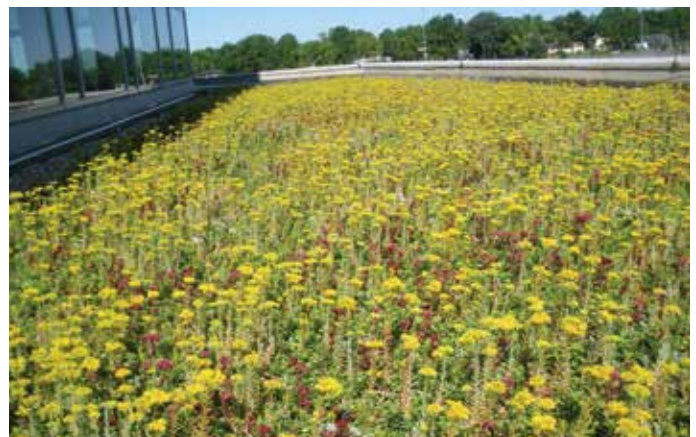
Fountainsdale Library - Bolingbrook, IL
