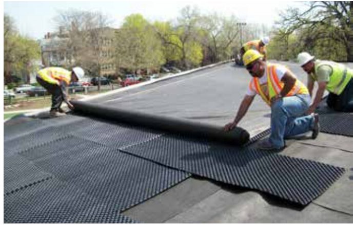
Systemfilter® installed to keep LiteTop® media out of Gardendrain®
