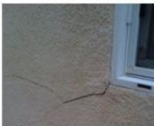
Fig. 1: Crack in exterior stucco
