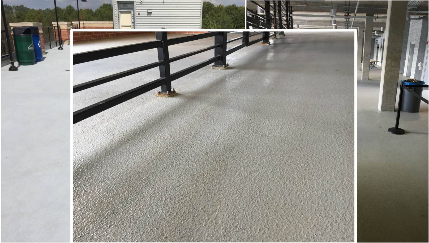
Stevenson University Stadium, Owing Mills MD Installed 2011, Pictures 2016
