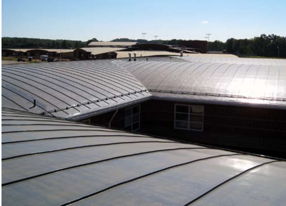
Complex angles come together atop the Sandy Valley Elementary School. The custom-colored lead grey roof has drawn favorable reviews from the community, and other school districts have sent representatives to Magnolia to view the roof.
